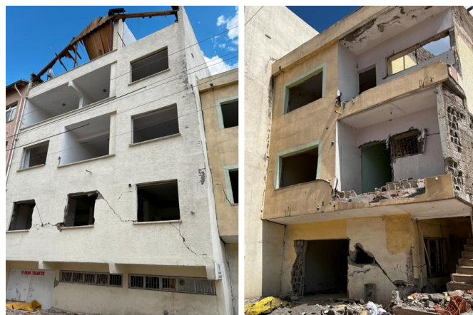
Fig. 10 Examples of damaged buildings
