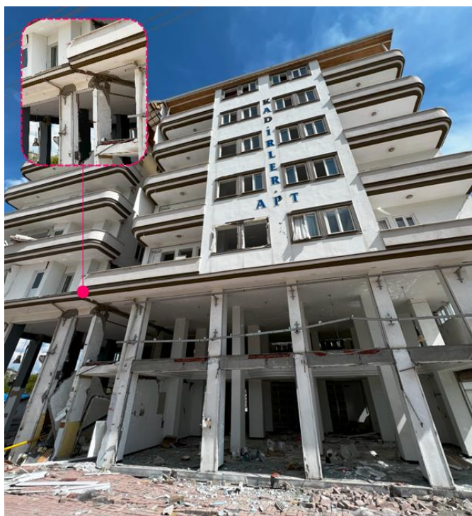
Fig. 8 Heavily damaged Kadirler Apartment
