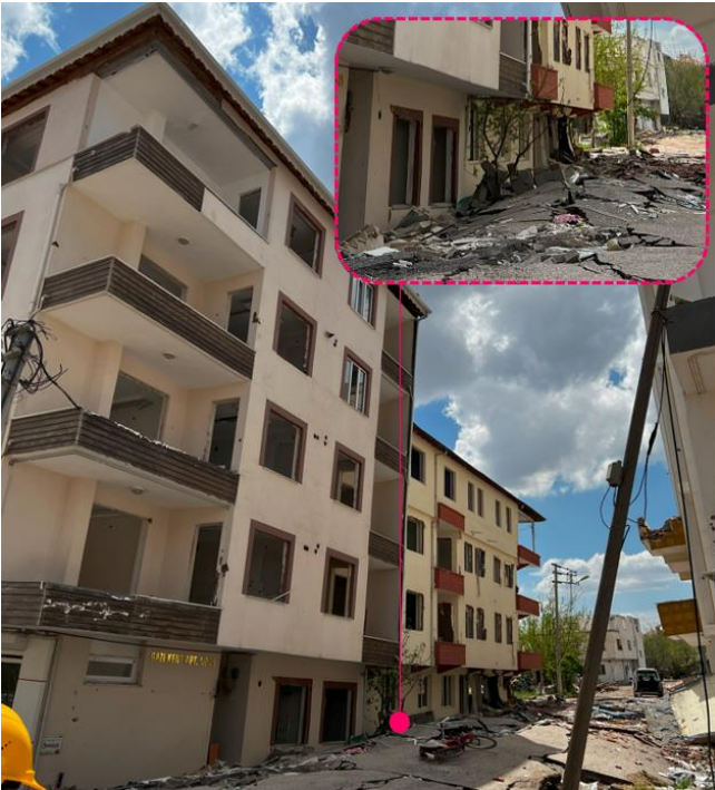
Fig. 4 Structures collapsing on the site
