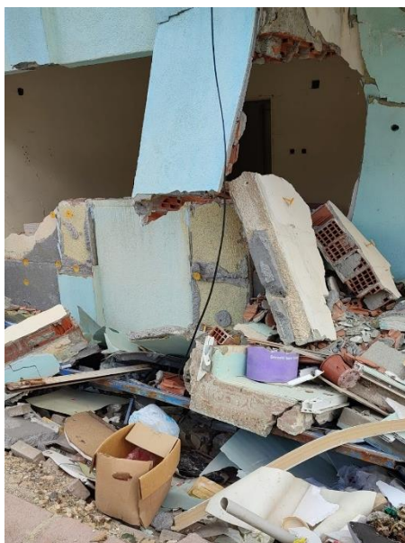
Fig. 9 Collapses caused by material use
