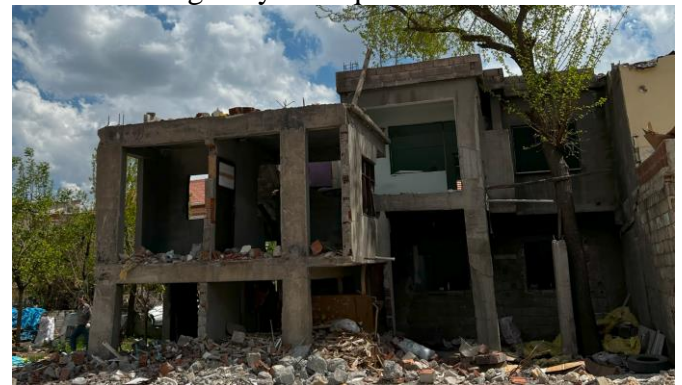
Fig. 7 Damaged building as a result of insufficient vibration, segregation and irregular load-bearing system etc.
